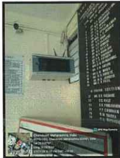
Outdoor Wi-Fi router in Entire Building through Cable connection
