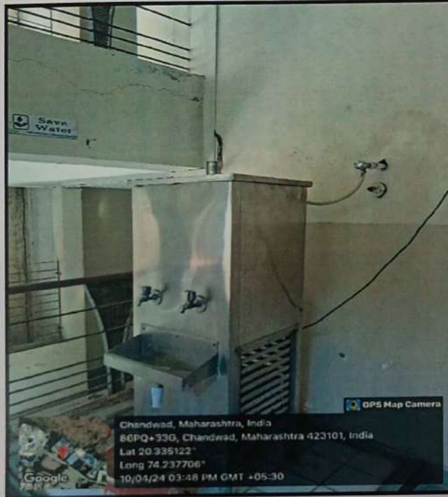
Water Cooler on each floor with save water sign boards
