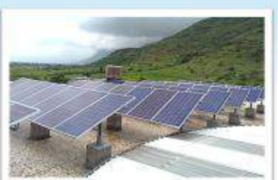
Solar PV System (400 KVA)
